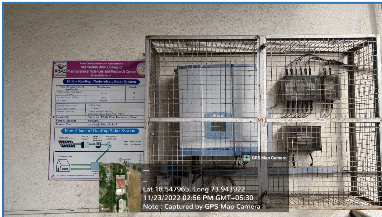
Solar System –Inverter
