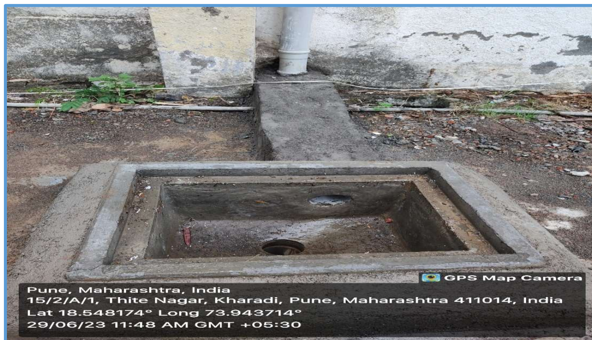
Rain water passes to bore well for recharge the groundwater level.
