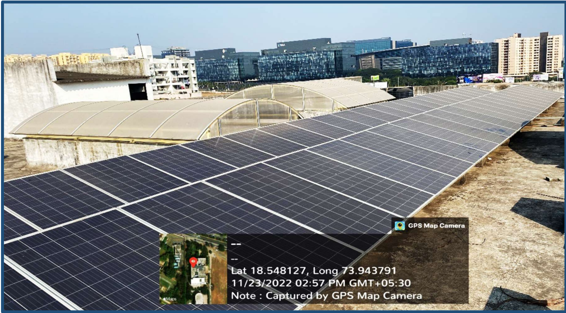
Rooftop Solar Photovoltaic System
